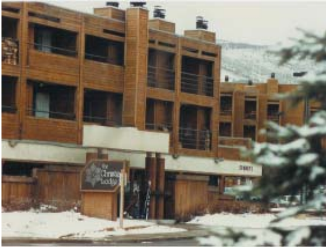
The original cedar siding aged quickly and was a maintenance headache.
